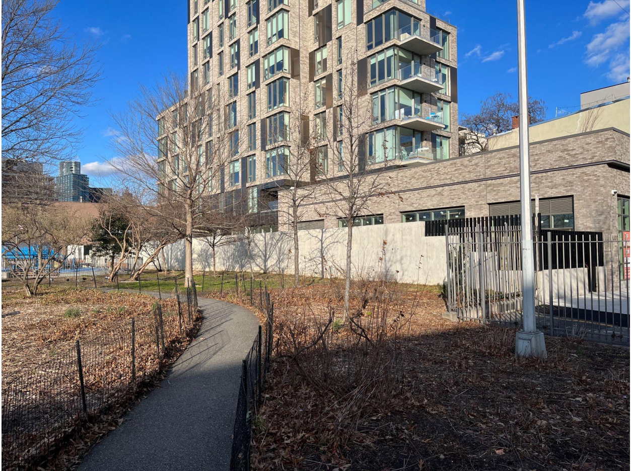
Figure 2 - Existing 8' high concrete border wall on the eastern border of WNYC Transmitter Park (ground elevation is 13').
